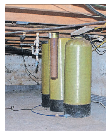
The filtration system Steven Vernik had installed in the home he owns in the Hartsville section of Warwick, after learning the private drinking water well was contaminated with high levels of PFAS. [WILLIAM THOMAS CAIN / CORRESPONDENT]
