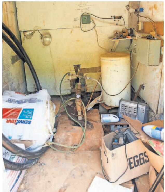
A small shed houses components of the water system for Coal Mountain, W.Va. Ravin Kenneda, 65, pours bleach into his community’s water every so often to keep it clean.
