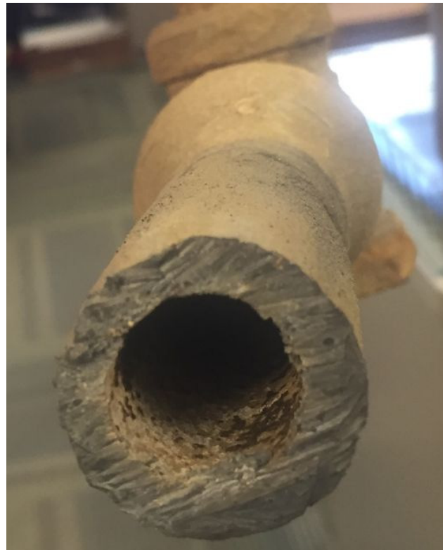
A lead service line removed from in front of a home in Southfield last year.
