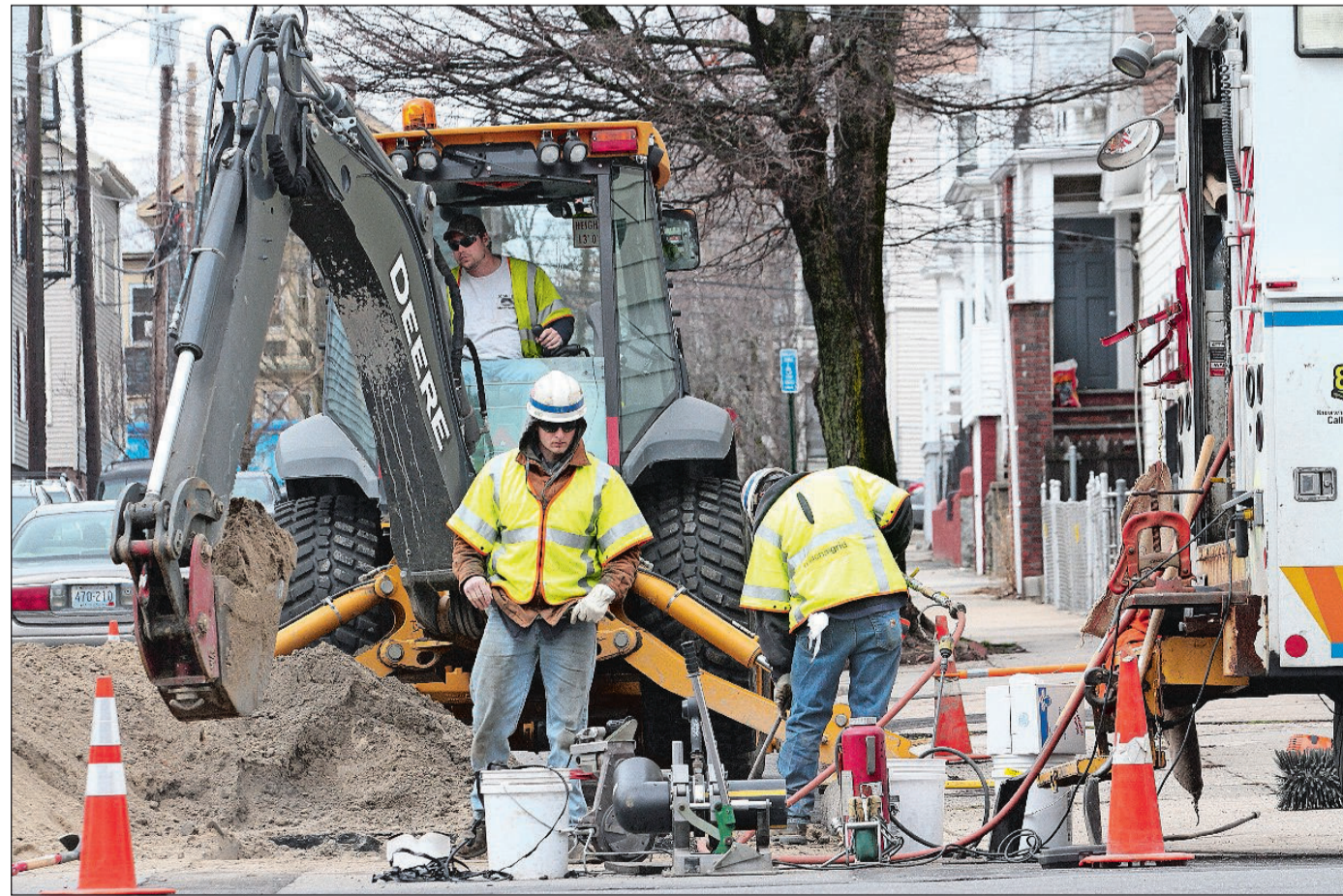
Gas line workers prepare to join pipes under Ives Street in Providence. National Grid will replace about 61 miles of pipes this year at a cost of about $100 million. [THE PROVIDENCE JOURNAL/BOB BREIDENBACH]
