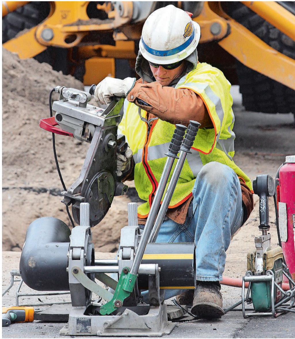
National Grid and private contractors connect businesses and residences near the corner of Ives and Fremont streets, in Providence, to a new gas main, replacing the old steel pipes with high-density plastic pipes. Rhode Island has an alarmingly high percentage of bare steel and iron pipes, both prone to leaks from corrosion and cracking. [THE PROVIDENCE JOURNAL/BOB BREIDENBACH]
