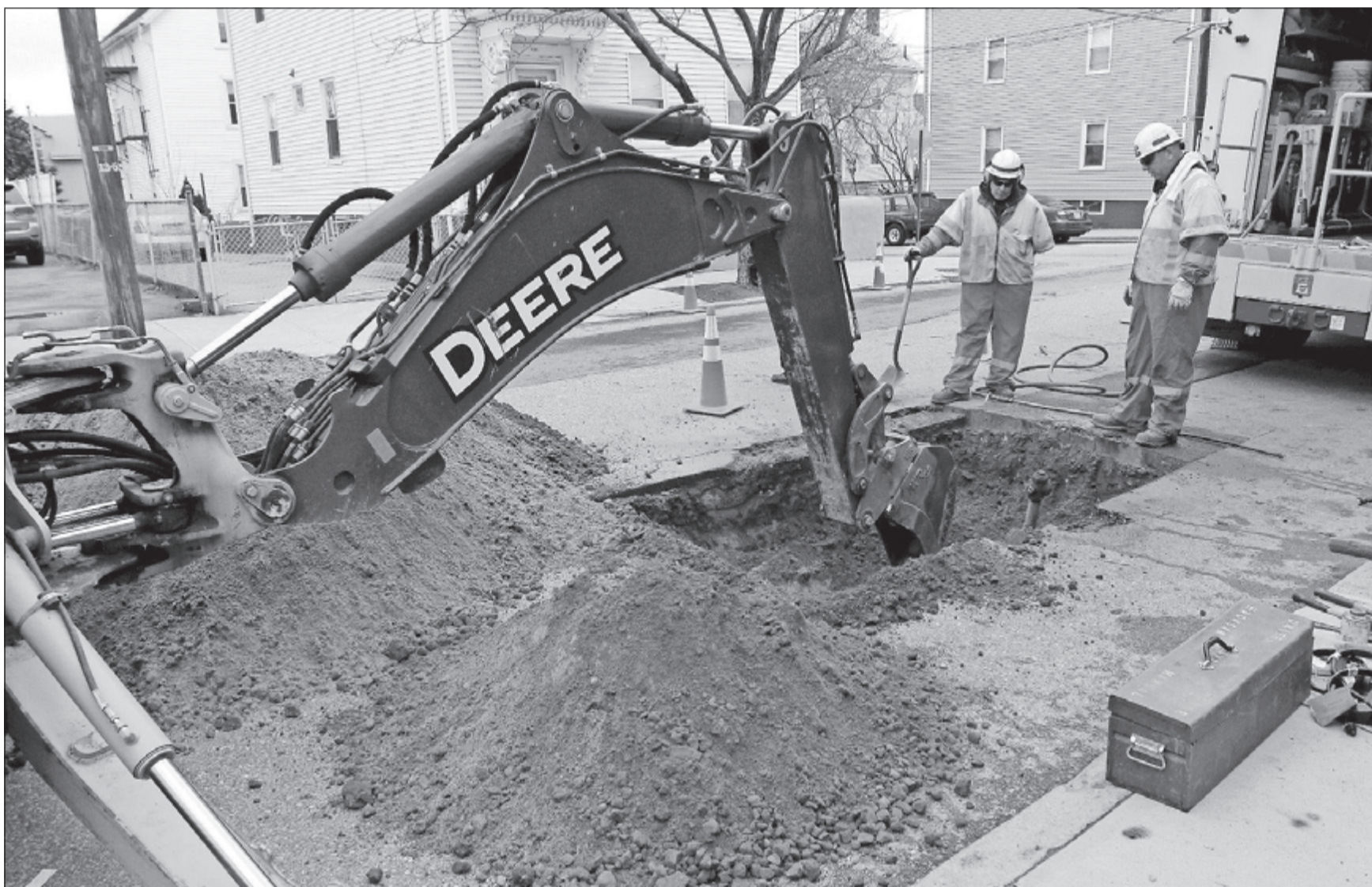
National Grid crews use a backhoe near Ives and Fremont streets, in Providence, to dig down to the existing gas pipe to allow a transfer to the newly installed pipe. [THE PROVIDENCE JOURNAL PHOTOS/BOB BREIDENBACH]
