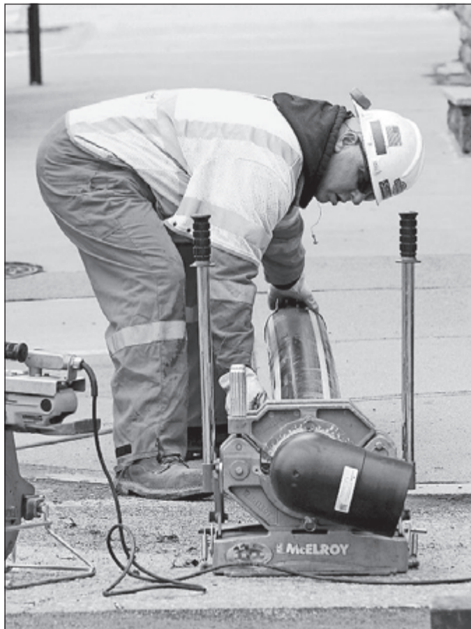
National Grid and private contractors work on connecting businesses and residences near the corner of Ives and Fremont streets to a new gas main, replacing the old steel pipes with high density plastic pipes.
