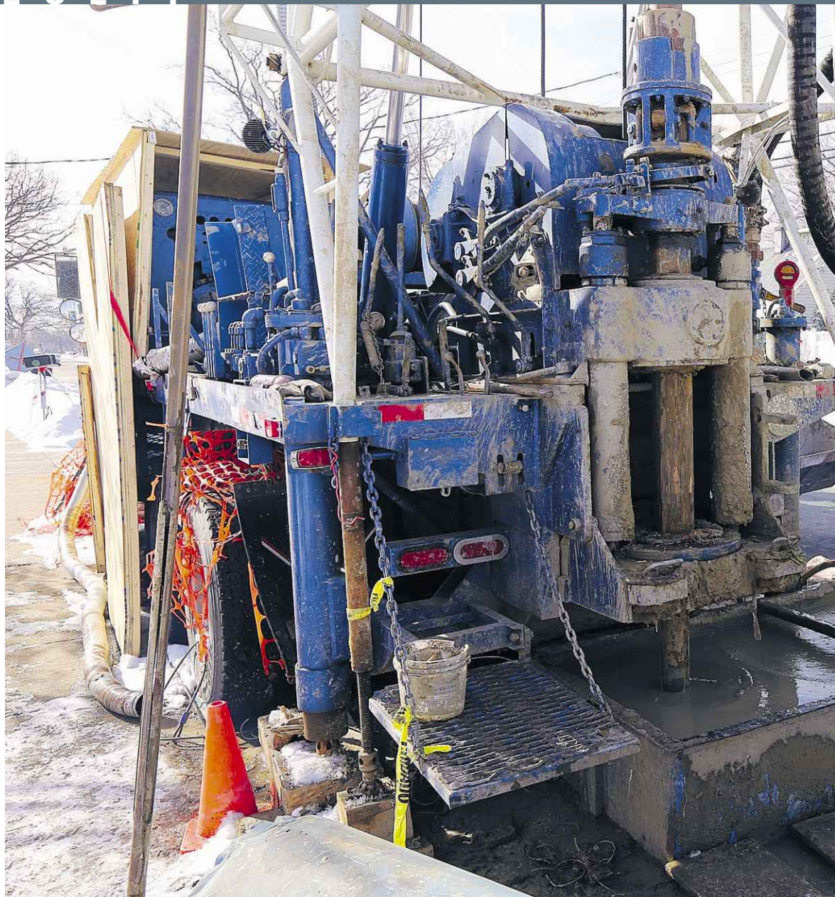
Northrop Grumman contractors drill to install a monitoring well at William Street and Broadway in
