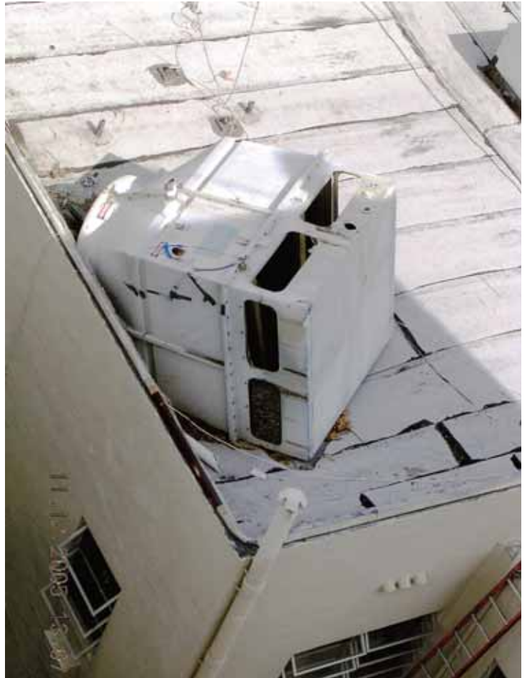
Part of an industrial-strength air conditioning unit that fell directly on top of reporter Dan Grech's condominium in Miami Beach during Hurricane Wilma just two months after Katrina in 2005, resulting in his forced hiatus for eighteen months after the city determined his home was unsafe to live in. PHOTO BY DAN GRECH
