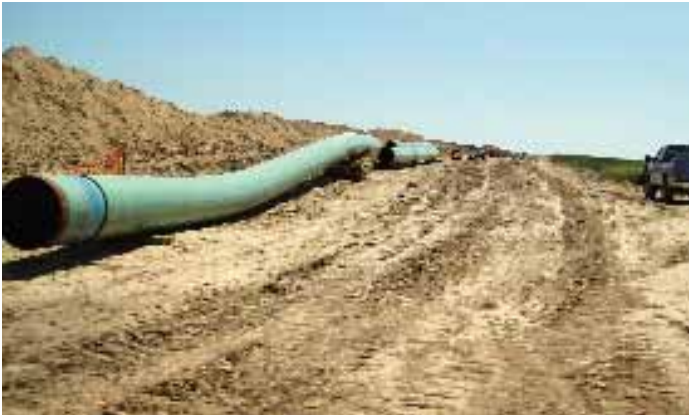
A portion of the Keystone Pipeline under construction near Swanton, Neb. in 2009. PHOTO: SHANNON PATRICK VIA FLICKR
