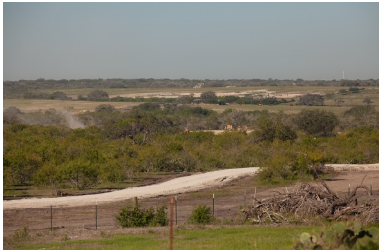
Clearing and grading take place for a new Marathon Oil fracking and well site in the Eagle Ford Shale, near Karnes City, Texas. (Lance Rosenfield/Prime)
